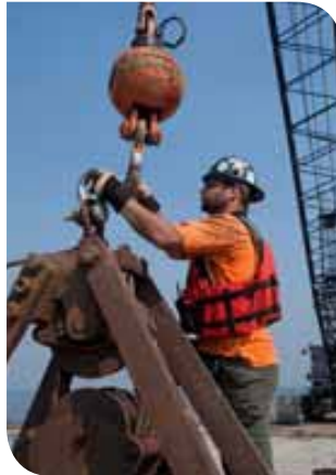
Geoff Tomczyk is among the almost 40 workers on the Deh Cho Bridge during the summer.
